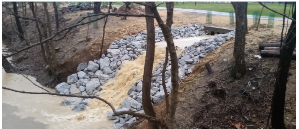
The top picture shows the condition of an outfall before the project began. The bottom picture shows the stormwater outfall stabilized in the same location during a large rain storm in 2017.
