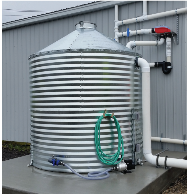
The Reading Municipal Garage Rainwater Collection and Reuse project turns rainwater runoff into a sustainable water source for use by the City of Reading
