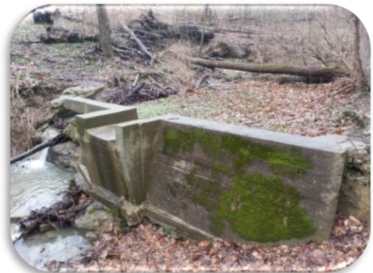
The existing dam in Cilley Creek causes severe erosion in the streambed and could release stored sediment should the dam fail
